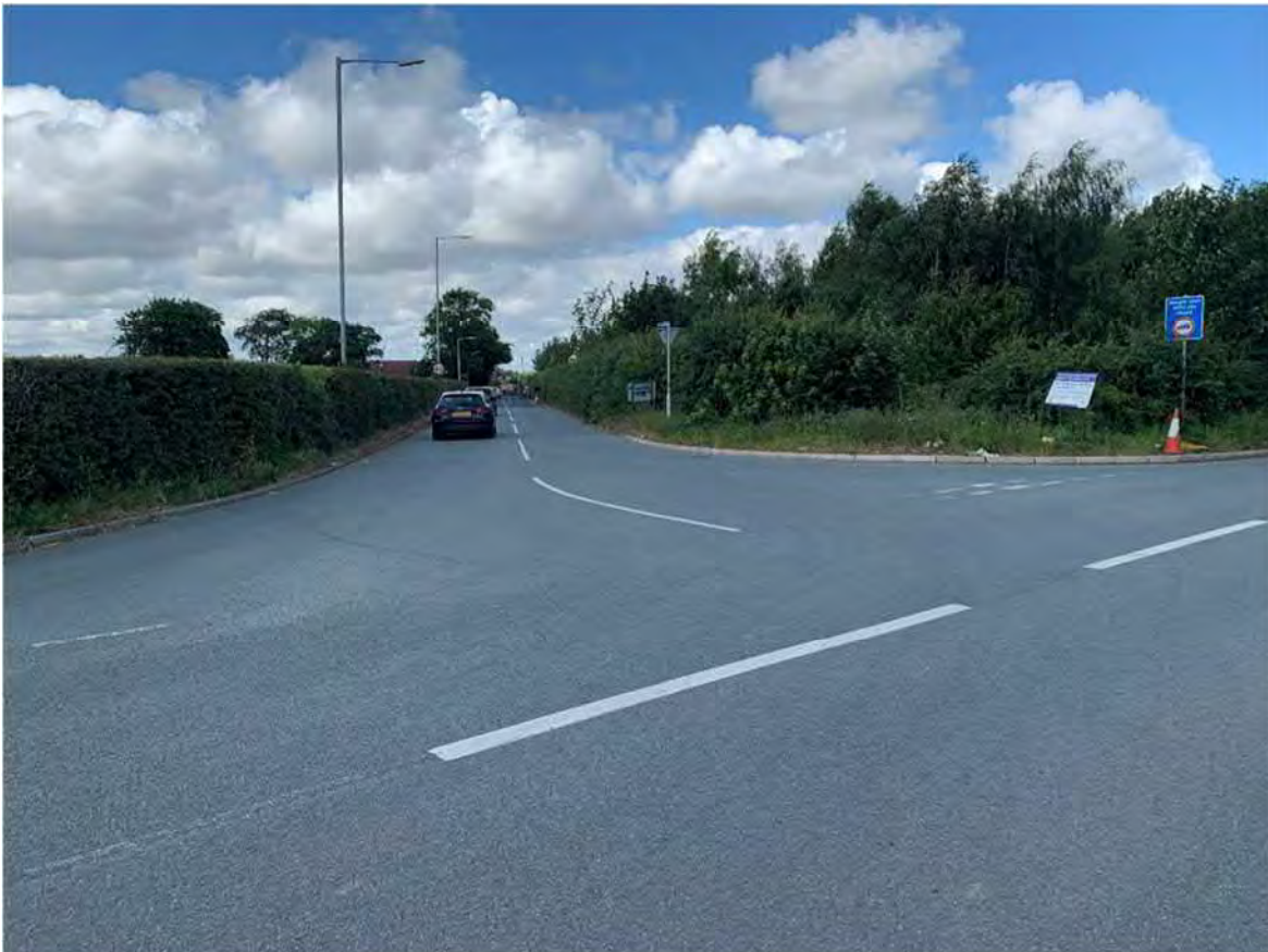
Figure 3-17 - Poor visibility with overgrown vegetation and tight bend
